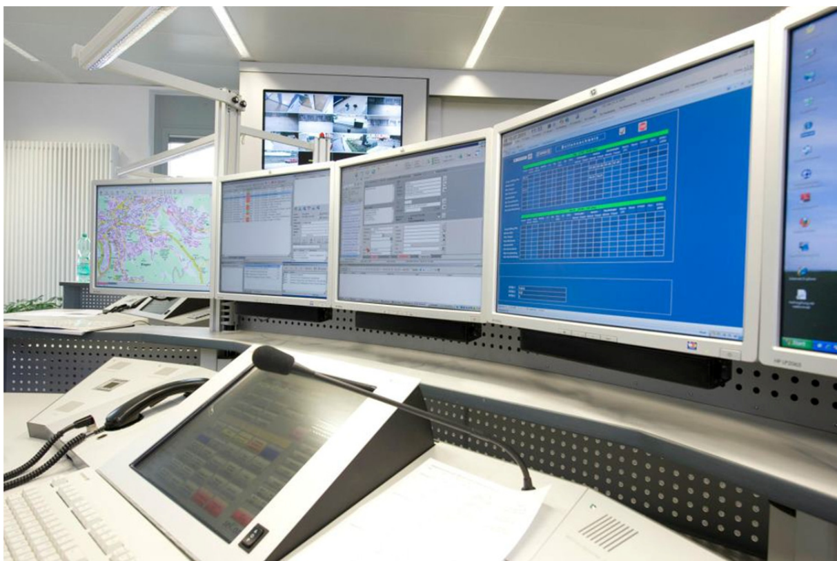
Figure 36: Work infrastructure in the control center
